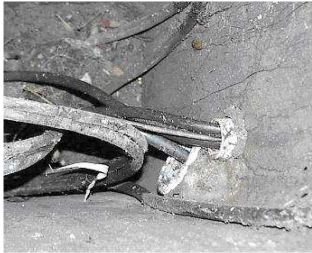
PLASTIC PIT AT CNR AJAX DR & BELINDA CR, WHEELERS HILL (27-SEP-2001) CLOSE UP VIEW OF CONDUIT EXITS AT RIGHT WITH MULTIPLE CABLES
