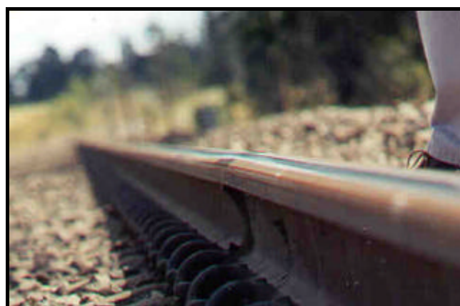
Figure 2 Example of Vertical Alignment Defect
