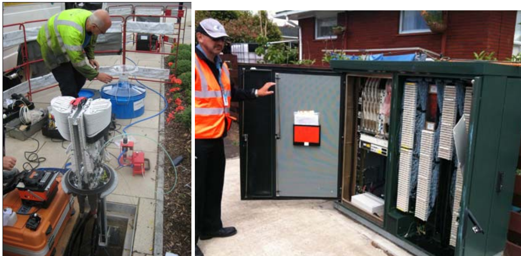
Figure 3.5: Underground enclosure (left) and street cabinet (right) for splitters [Source: Analysys Mason]
